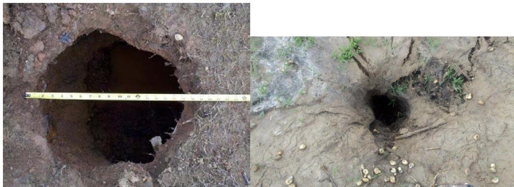
A sinkhole identified in the HOA's 2012 consultant report (left). It's almost 18" wide. At right, a sinkhole identified in 2011; it is only 5 inches wide.
