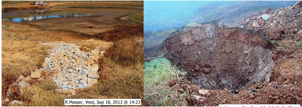
Lake view just before work began on sinkholes (left). Excavation of sinkhole during repair work (right).
