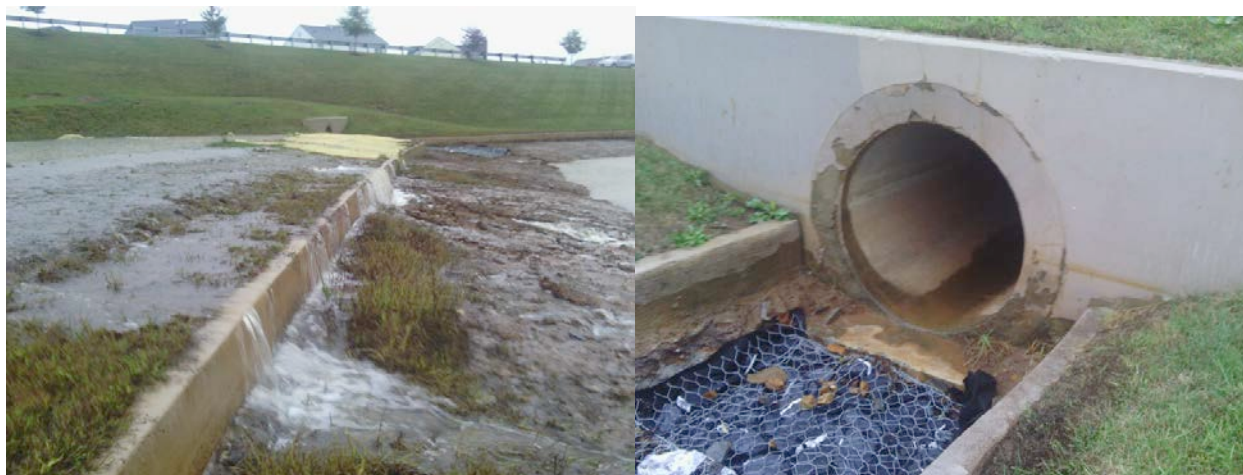
FIGURE 2—Overflowing forebay near the clubhouse, October 11, 2013. Meanwhile the large outfall pipe near the clubhouse discharged almost no water to the lake.
