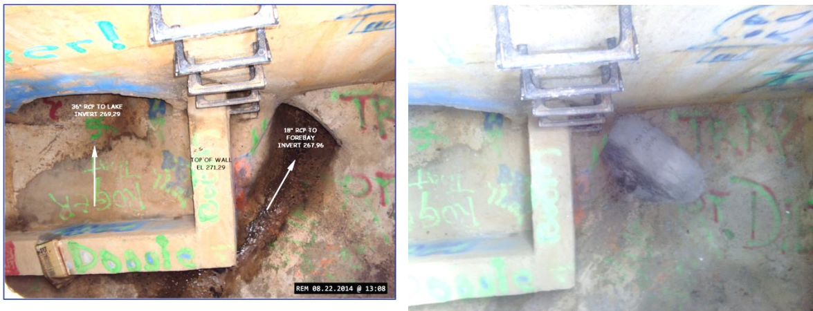
FIGURE 4: The “splitter” in these two images sends early stormwater to the forebay through the 18 inch pipe on the right of the image. As larger volumes flow to the splitter, water is supposed to back up and spill to the 36 in pipe on the left side leading to the lake. However, the 18 inch pipe was too large for its intended purpose and water rarely went to the lake. The image on the right shows the 18” opening restricted to only a 4” opening. The other two splitters should receive the same modification.
