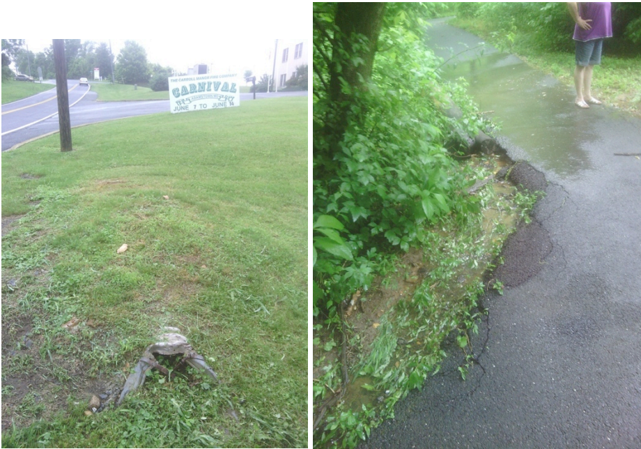
FIGURE 8: This drain pipe near Ballenger Creek Pike discharges to the walking path (left). The water damage to the walking path is evident in the image on the right.
