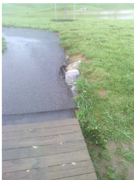
FIGURE 7: Erosion near bridge.
