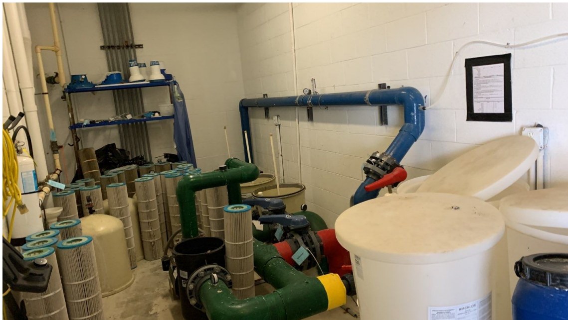
General Site - Pool, Equipment
