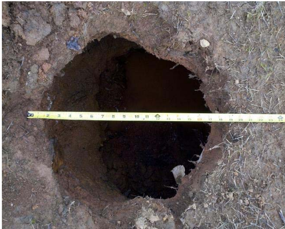
Photograph 2: View of sinkhole between the pool and retaining wall.
