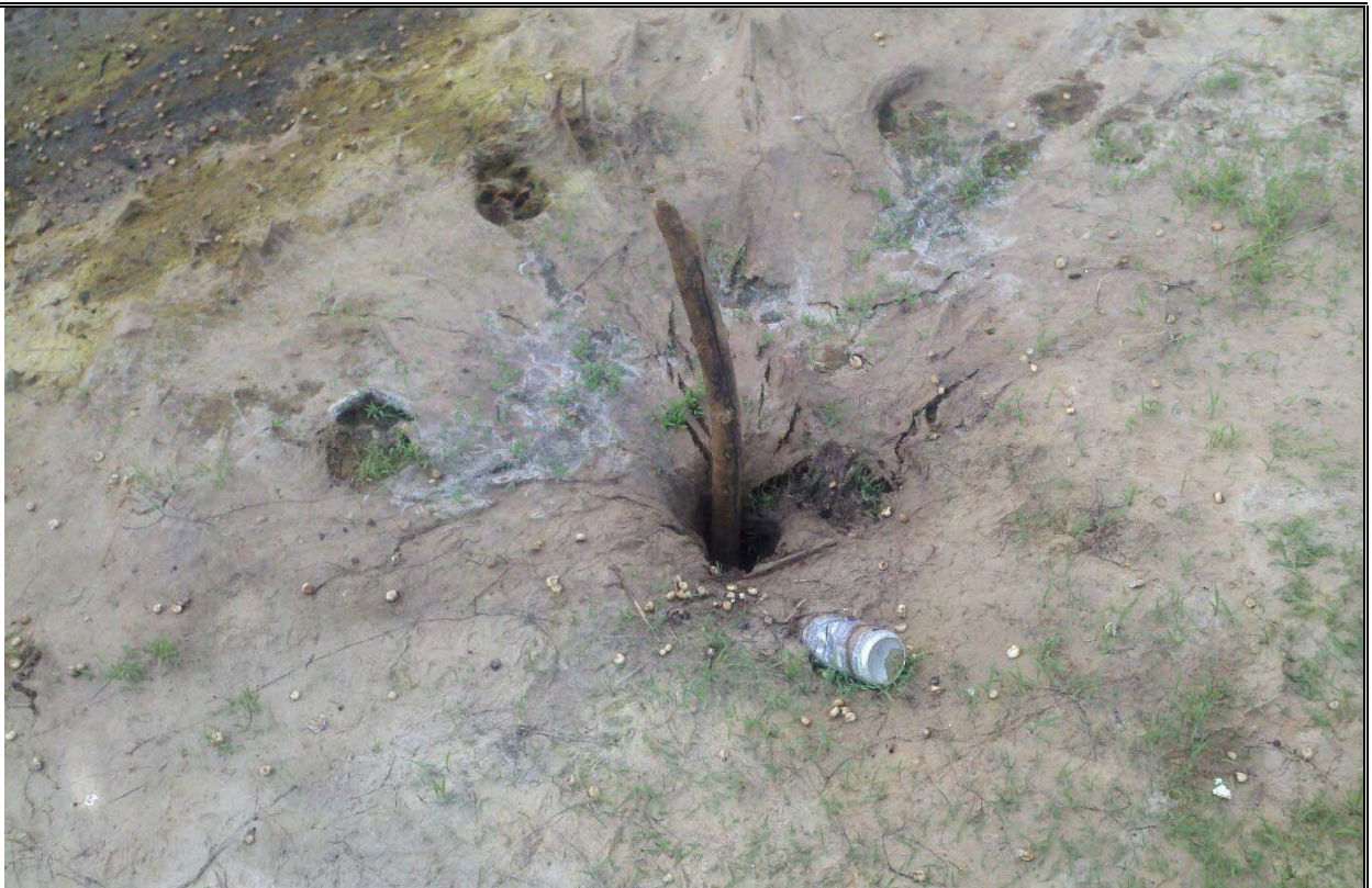
Photograph 4: Sinkhole in between the pool and the retaining wall.
